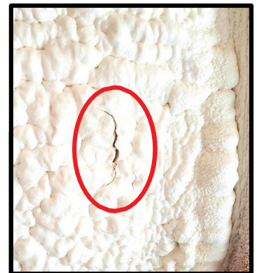
2.0 MAX sprayed at 3.5” in August Initial cracking begins to occur in Nov at first exposure to sub-freezing temperatures.
